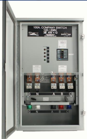
Sub Distribution Board
