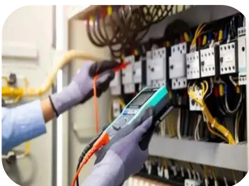
Installation & Testing Panel
